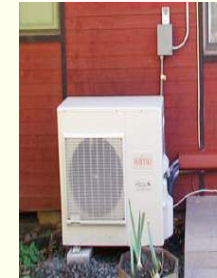
Ductless Cooling Commercial
