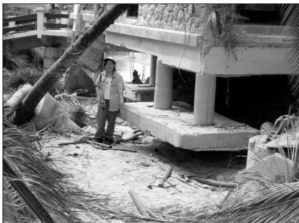
FIGURE 4 Example of scour below a shallow footing in the Khao Lak area. The building was several hundred meters from the ocean.
