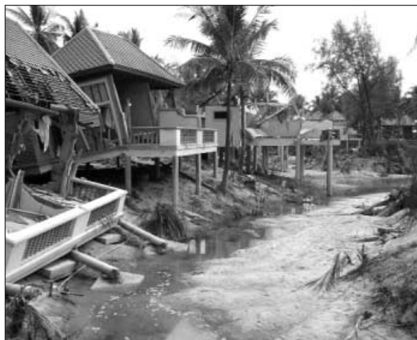
FIGURE 5 Structural damage at a Khao Lak resort, illustrating both foundation failure due to scour and direct wave impact. This level of devastation was observed in many areas.
