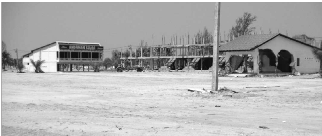
FIGURE 6 Buildings at Khao Lak. The wave came from the left and broke through the masonry walls of the building on the right. The Andaman Scuba building was relatively untouched by the wave because of the large number of display windows that broke out and the streamlined footprint of the trapezoid-shaped building.
