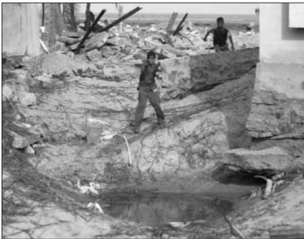
FIGURE 6 Typical damage from scouring at the foundation of a building on the east coast of Sri Lanka.
