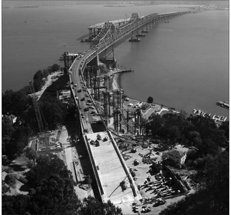
FIGURE 2 Aerial view of the east span of the San Francisco-Oakland Bay Bridge, Labor Day 2007, with the replacement deck piece newly installed. Demolishing the old viaduct sections and moving the prefabricated section into place was accomplished in 70 hours—11 hours ahead of schedule. (Photo: Barrie Rokeach, Aerial/Terrestrial Photography.)
