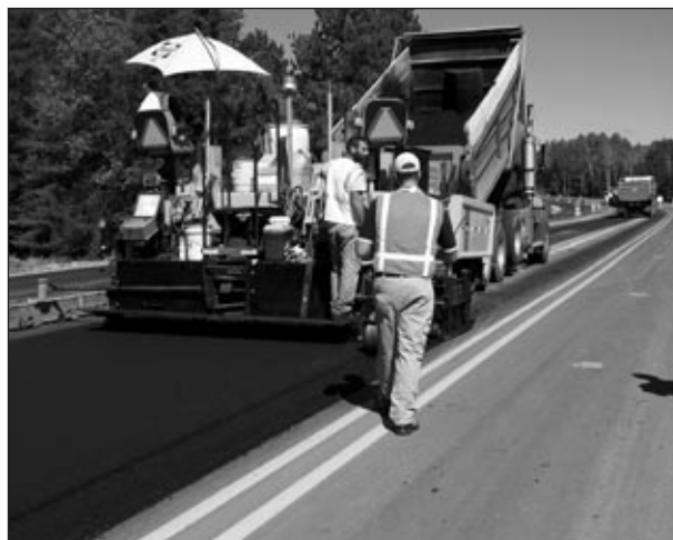
FIGURE 1 Superpave application on Michigan State Route 95, near Iron Mountain. The Superpave system, which matches the combinations of asphalt binder and crushed stone to the climatic and traffic conditions on specific highways, was developed under the National Research Council–managed Strategic Highway Research Program and is in use in every state. (Photo: Larry L. Michael.)
