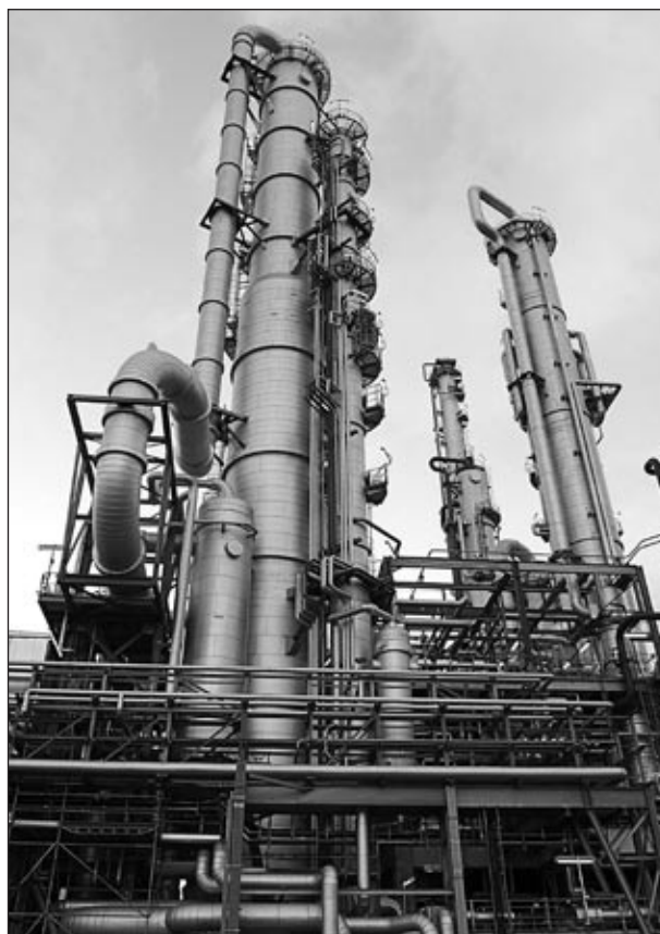
FIGURE 1 The new HPO plant at the BASF site in Antwerp, Belgium, completed the startup phase in 2009. With a new process for producing propylene oxide jointly developed by BASF and Dow, wastewater is reduced by up to 80 percent, and energy use is reduced by 35 percent compared to conventional processes. Source: BASF.
